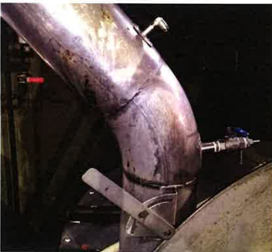
104: Separator Feed Tank Ports 14 – 14a
