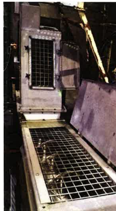
107: Drainer Conveyor Hatch
