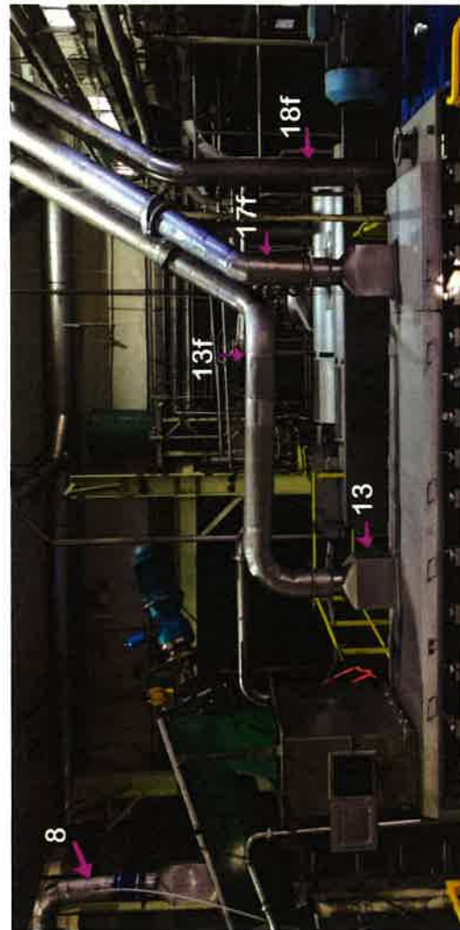
112: Press Extraction Ducts
