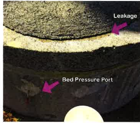
105: Covered Biofilter Sump
