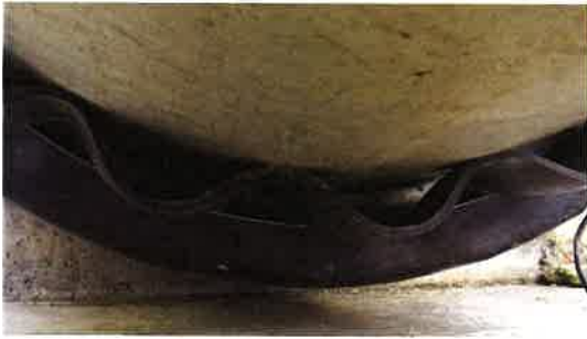
102: Fan 14.1 Discharge Duct Seal
