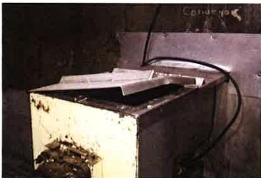
110: End of Press-Decanter Solids Conveyor in Dry Area
