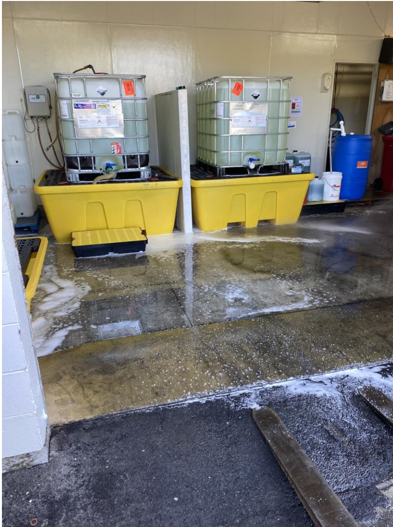
Figure 4: Hazardous substances within bunded area and connected to tradewaste/waste water system.
