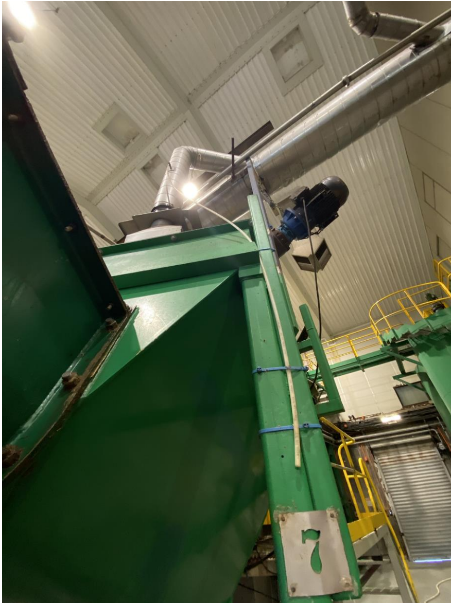
Figure 2: Port 7 extraction testing pipe on 'wet' side of rendering process.
