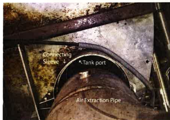
125: Decanter Feed Tank 2.11 air extraction duct
