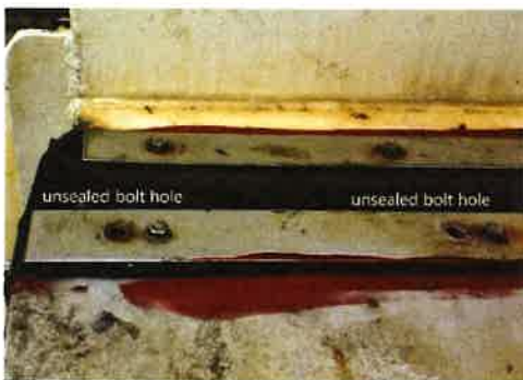
102: Fan 14.1 unsealed old open bolt holes
