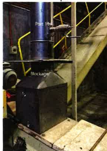
119: Port 15 - Driers Discharge Conveyor
