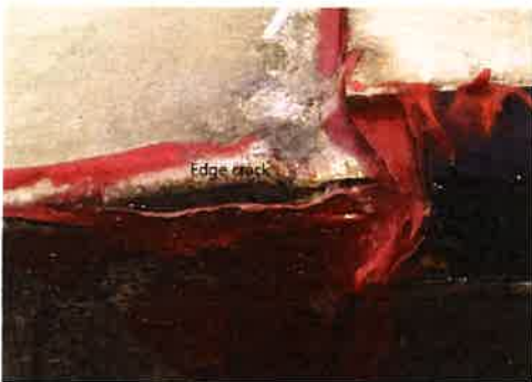
103: Fan 14.1 outlet transition duct cracking
