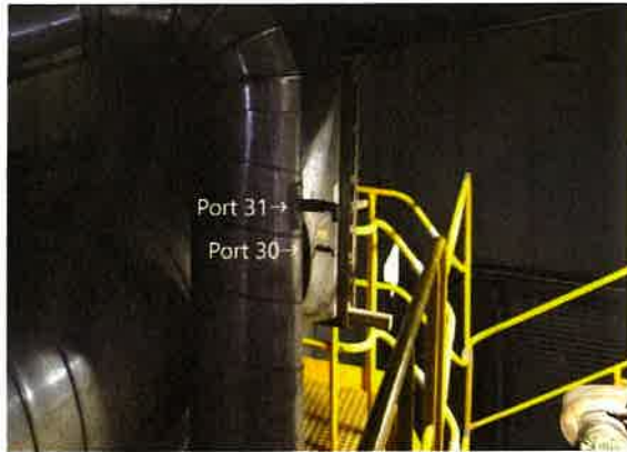
120: Ports 30 and 31 – Dryside Extraction Louvre
