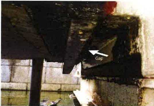
101: Fan 14.1 outlet transition duct seal leak
