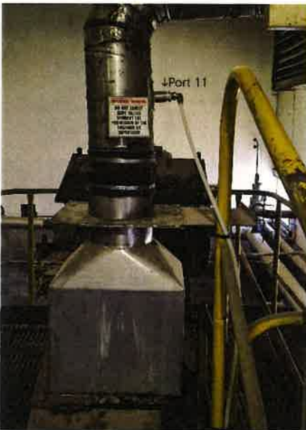
115: Port 11 – Inlet conveyor to Driers
