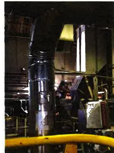
106: Port 4 - Preheater Discharge
